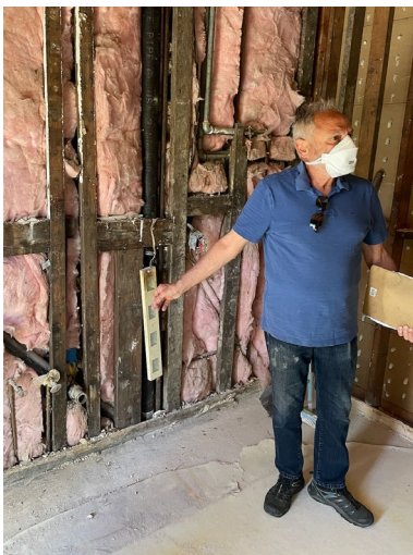
AV Maintenance Manager Sal Romano explains plumbing issues to members in June. Photo by Madeline Marrow.
